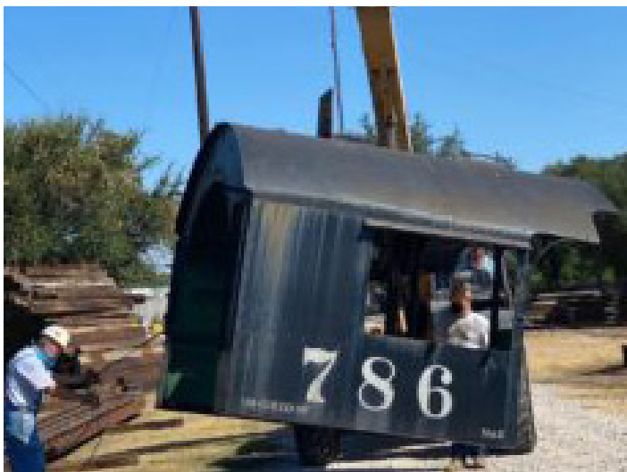
A crane lift brought 786's cab from the back of the ASTA yard to a location where it can be cleaned, repaired, painted and relettered before resuming its position of honor on the engine.
